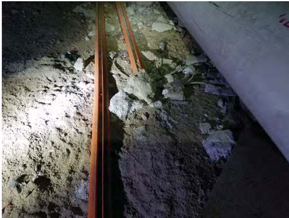
Example of thermal system insulation debris in Building 3
