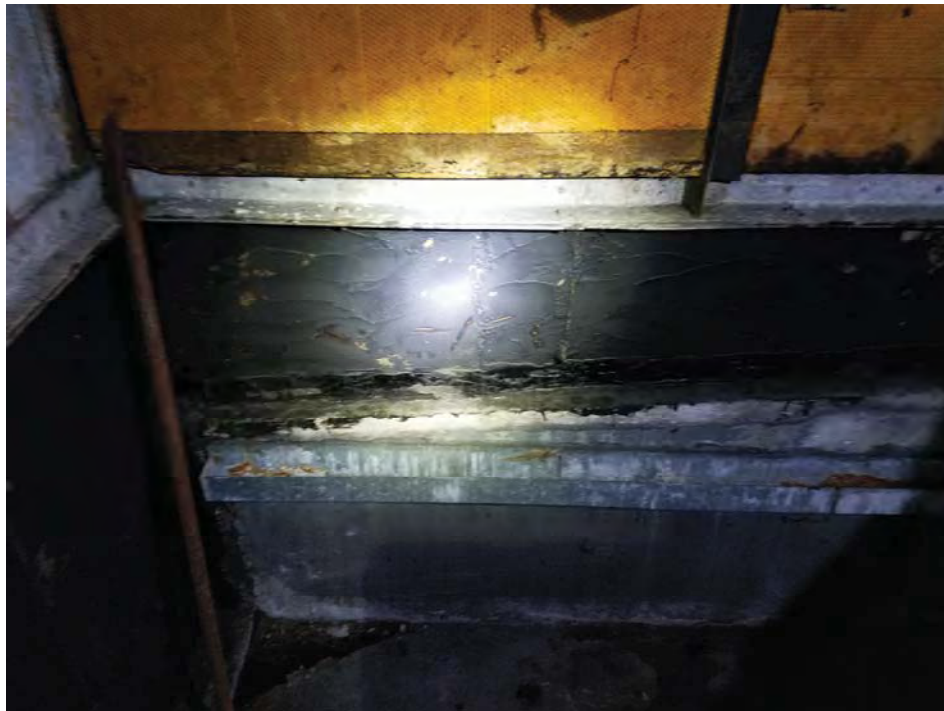
Example of black mastic on AC units in Building 3
