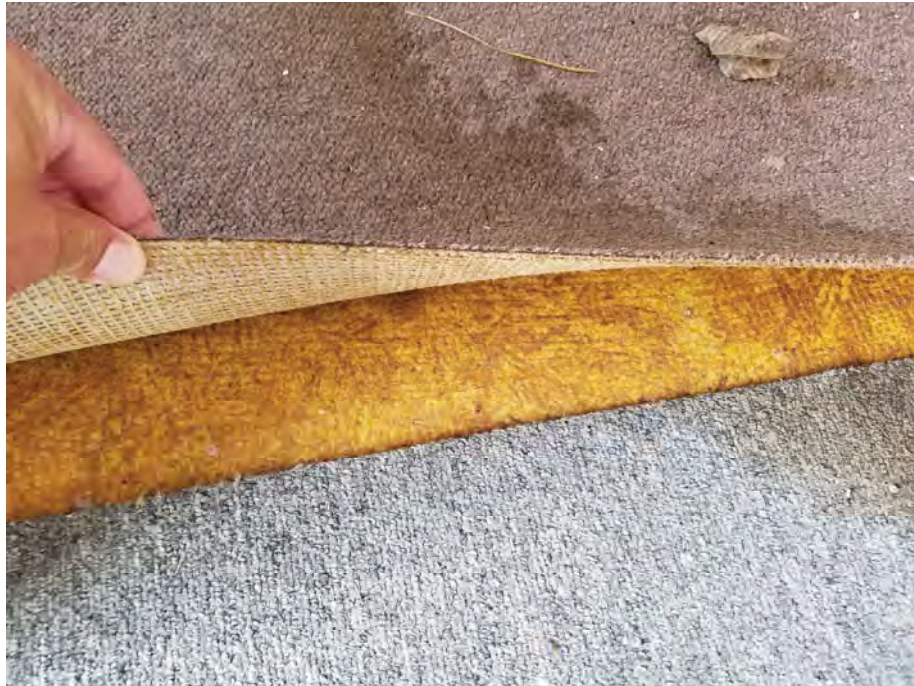
Example of asbestos-containing vinyl sheet flooring under carpet in Building 2
